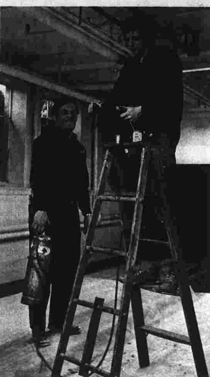
Repairing Community Y Donald Ryder, left, and Donald Ryder Jr., right, work on repairs to water pipes in the Community Y building on N. Main St. The pipes in the building are being replaced, and the work is being done by D & R Plumbing Co., Inc. of Rockville. (Herald photo by Pinto)
